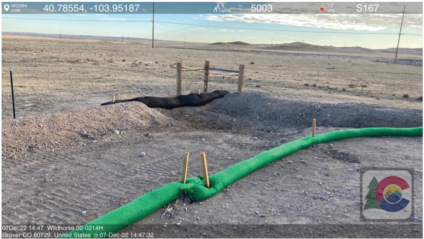
Excavation backfilled and stormwater BMPs improperly installed.
