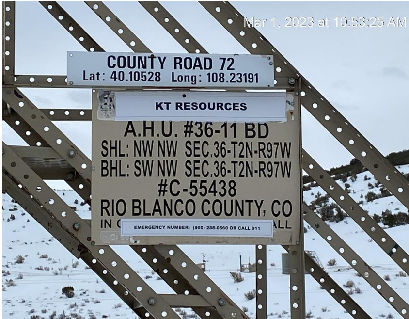
Sign at tank battery
