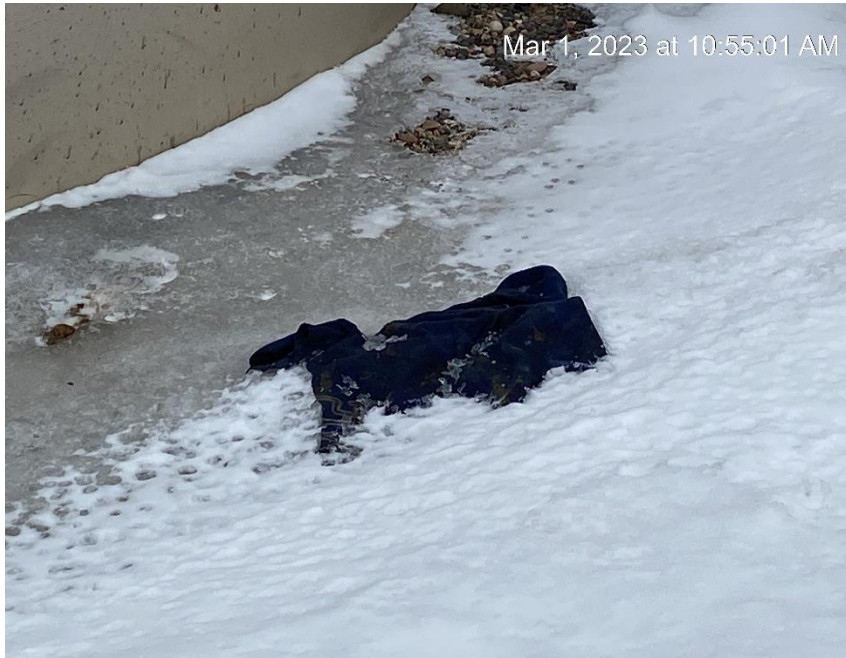
Debris inside tank battery
