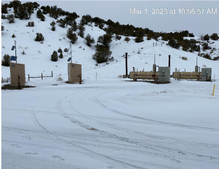
Separators and meter runs
