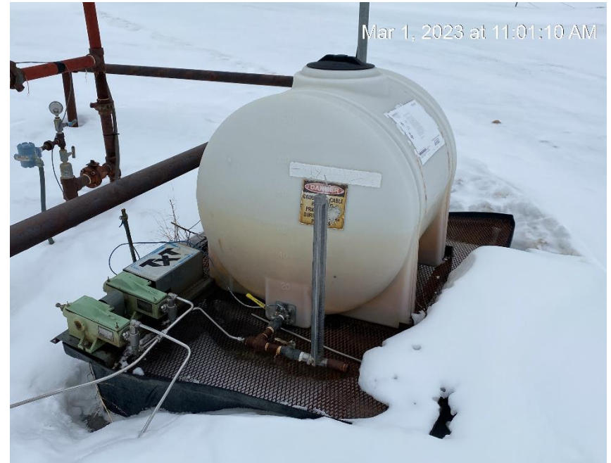
Tank label illegible. No placard label.
