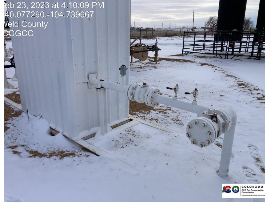
Pic 6 gas meter run valve appears to be open
