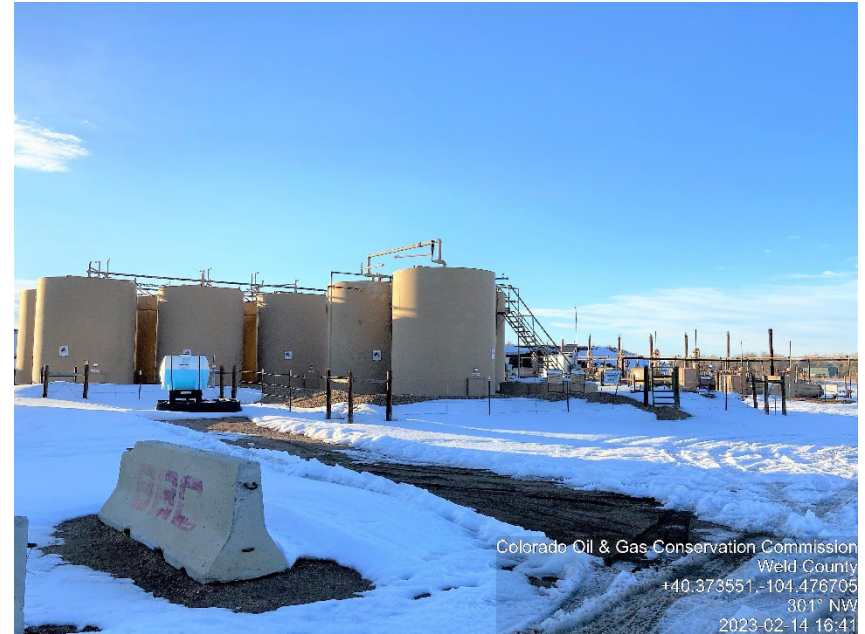
Photo #2 Peterson CX GH 30-14D, 30-41D, 30-26D, 30-40D, 30-28D, Peterson 30-31, 30-32, 30-41, 30-42, 30-51. Battery site Inactive | Shut-down Equipment documented: Loc. # 430376
