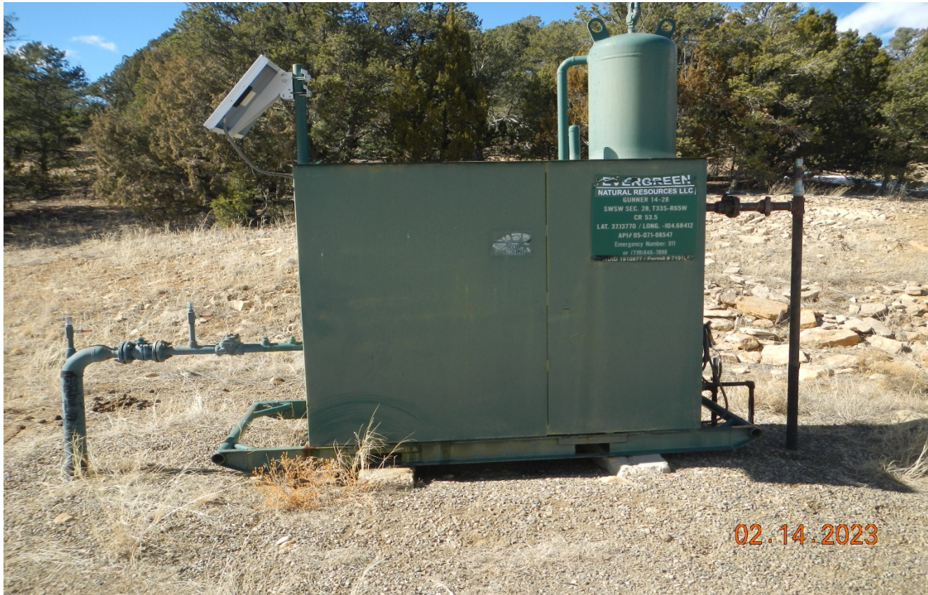
Photo 3. Sign posted at meter shed. Operator name is peeling off on the sign.
