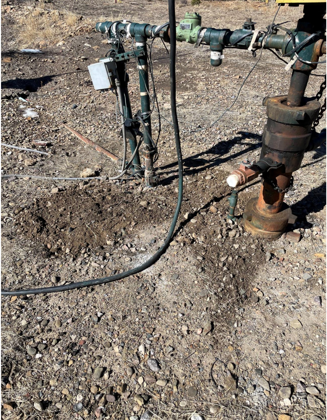
Conducted Maintenance on equipment, cleaned up stained material and reviewed self-inspection to comply with Rule 1002,(2)D. (Repaired Leaking Equipment)
