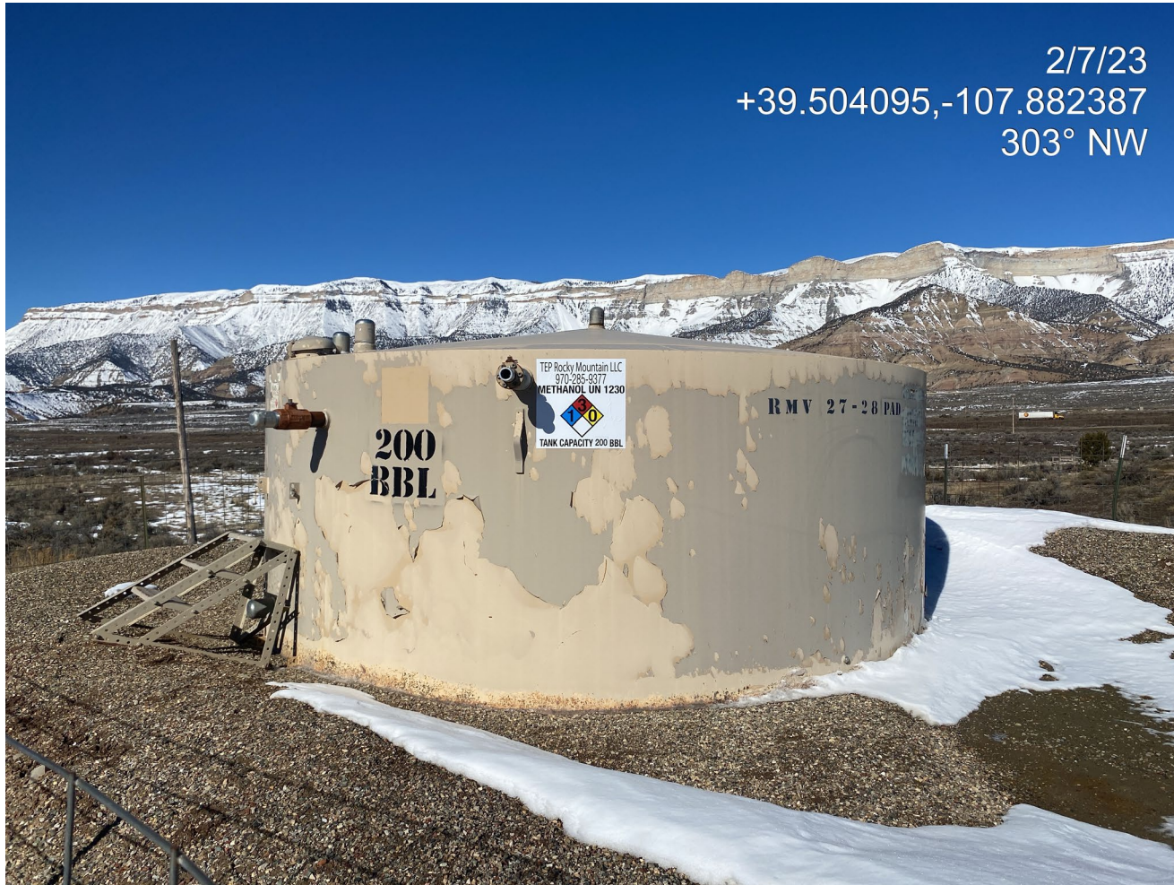
Photo 2. Photo shows a newly applied label on a methanol tank.
