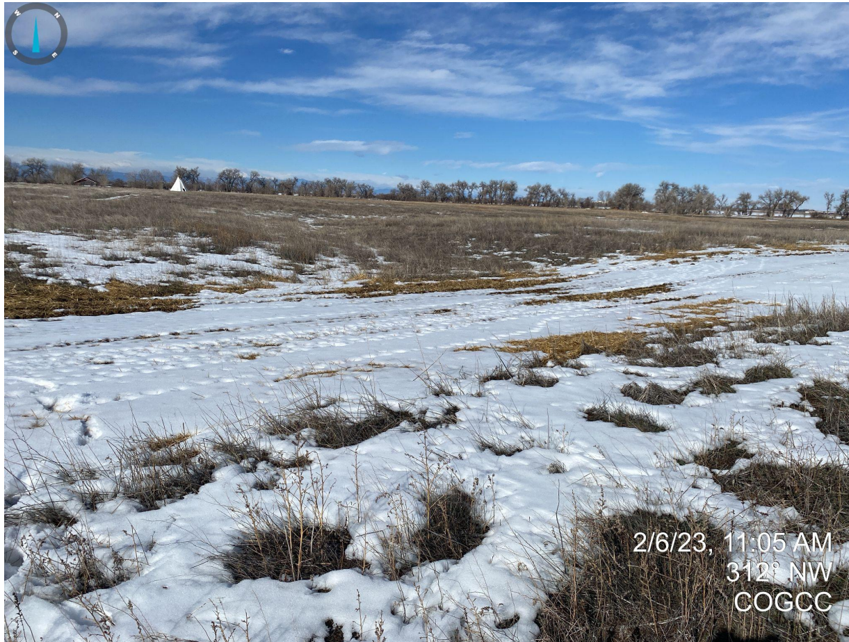
Photo 2. Facing northwest from the former access road. It appears the operator has performed the corrective action and recontoured the former access road to reflect natural/reference area topography and performed revegetation activities.
