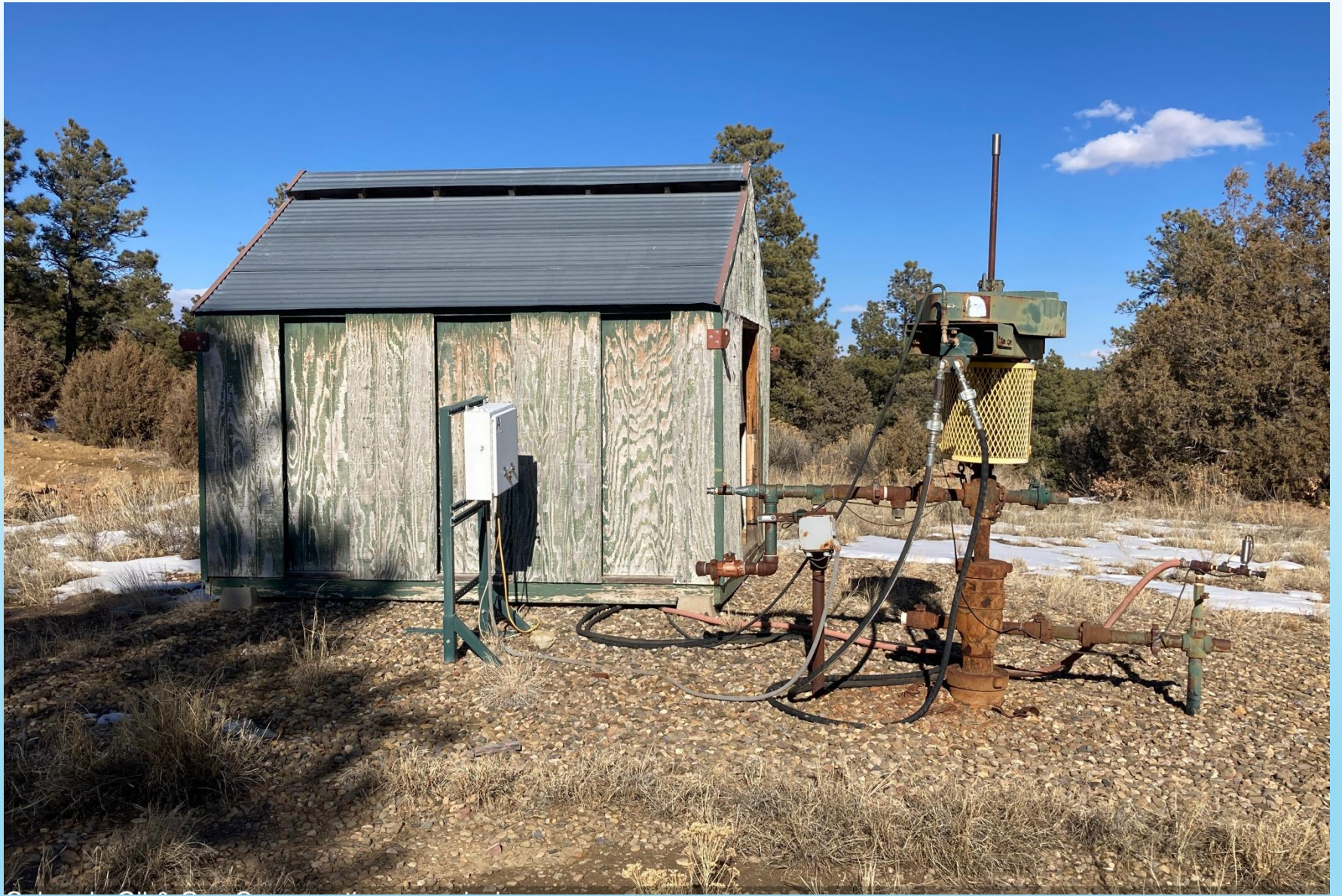
PHOTO 3: ORIGINAL WELLHEAD AND EQUIPMENT
