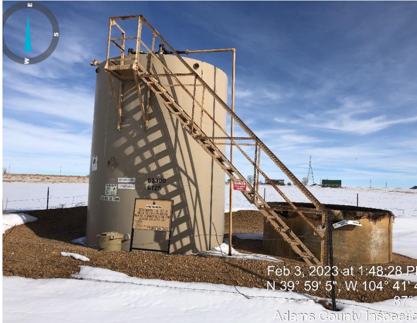
Photo# 1 Crude and P/W tanks.
