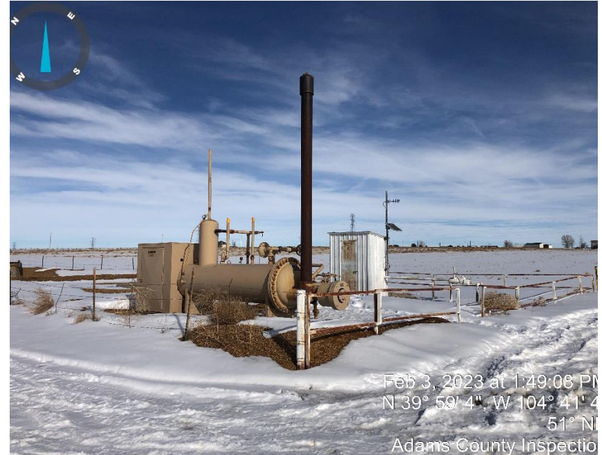
Photo# 2 Meter house and Separator.
