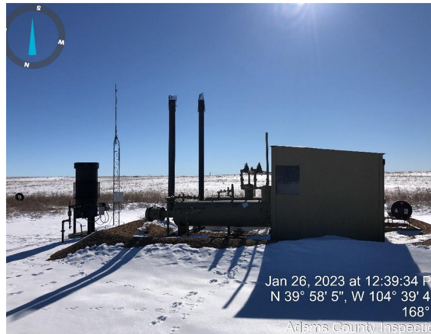
Photo# 2 Separators, ECD & RTV.
