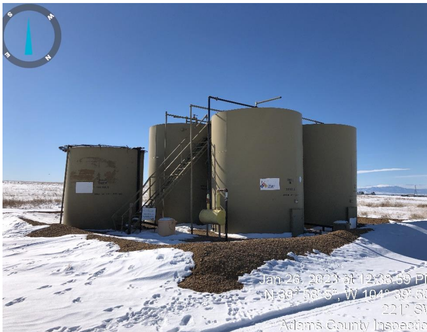
Photo# 1 Crude tanks & P/W tank.
