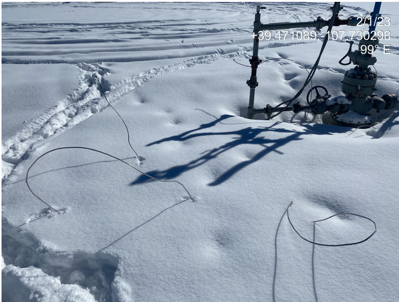
Photo 2. Photo shows old injection line equipment/debris.
