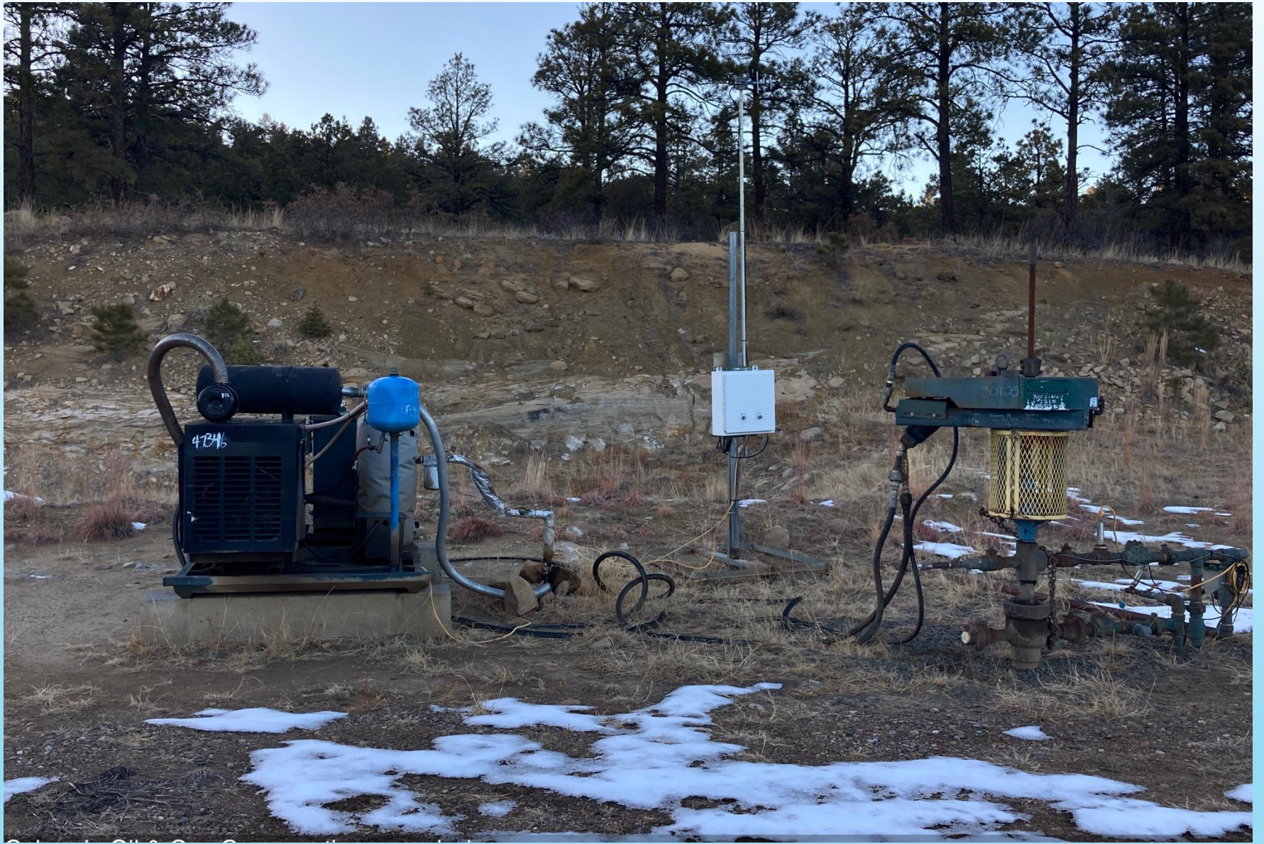
PHOTO 3: ORIG. WELLHEAD AND EQUIPMENT
