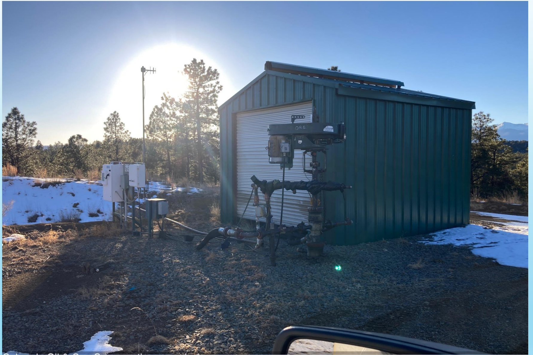
PHOTO 3: ORIG. WELLHEAD AND EQUIPMENT
