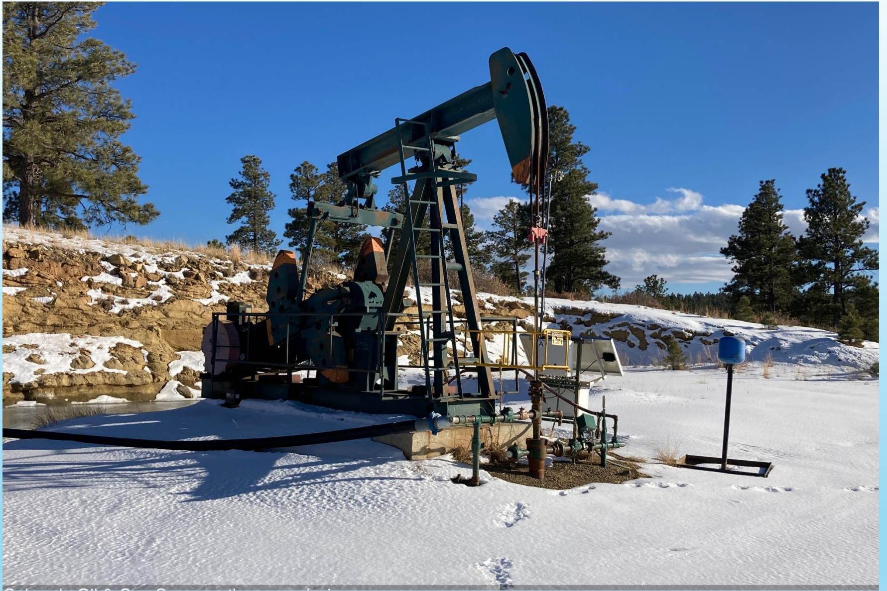
PHOTO 3: WELLHEAD AND EQUIPMENT
