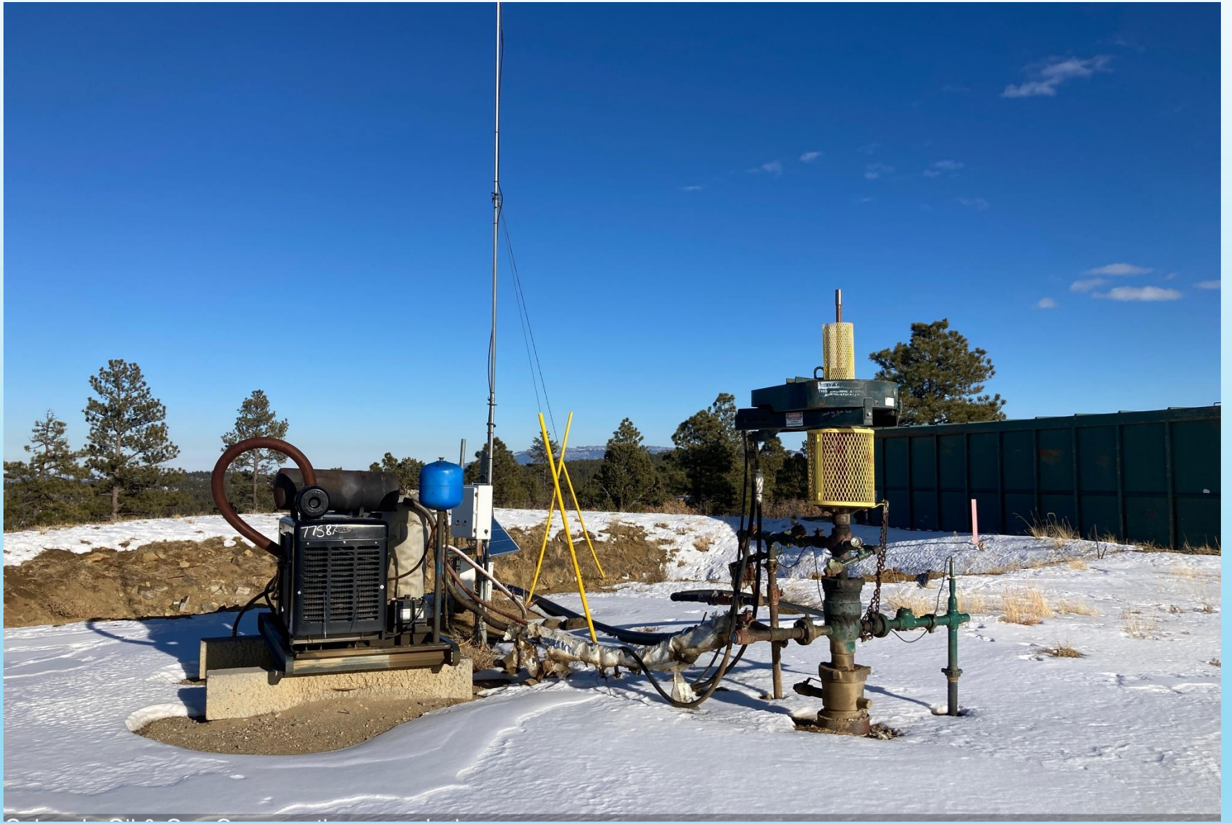
PHOTO 3: KV WELLHEAD AND EQUIPMENT
