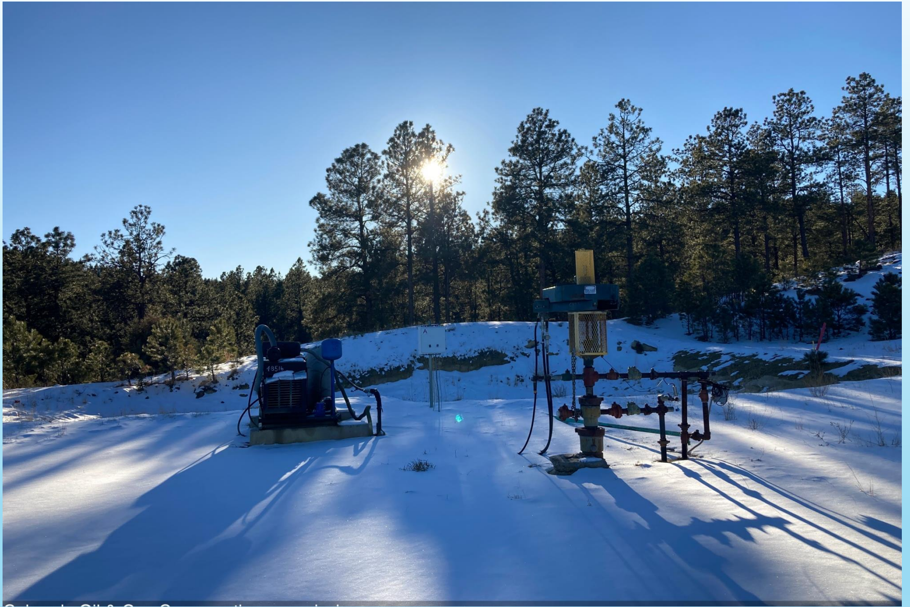
PHOTO 3: WELLHEAD AND EQUIPMENT
