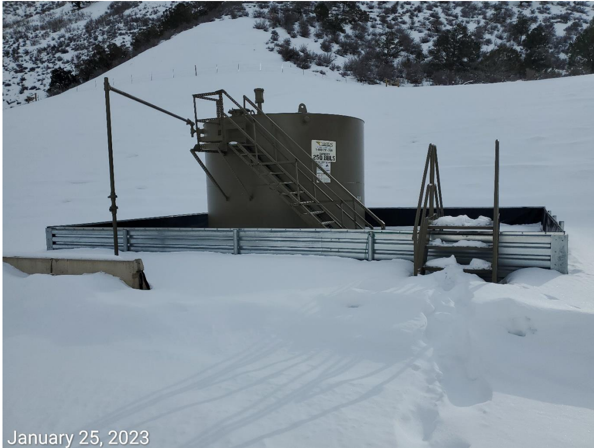
Photo 4: Photo shows signage missing from the tank battery.
