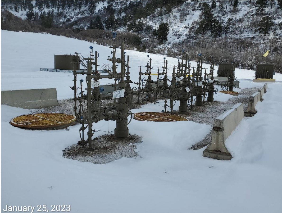
Photo 3: Photo of wells on Location. Photo also shows three conductor settings remaining on the Location- conductors associated with expired well permits, and require removal.
