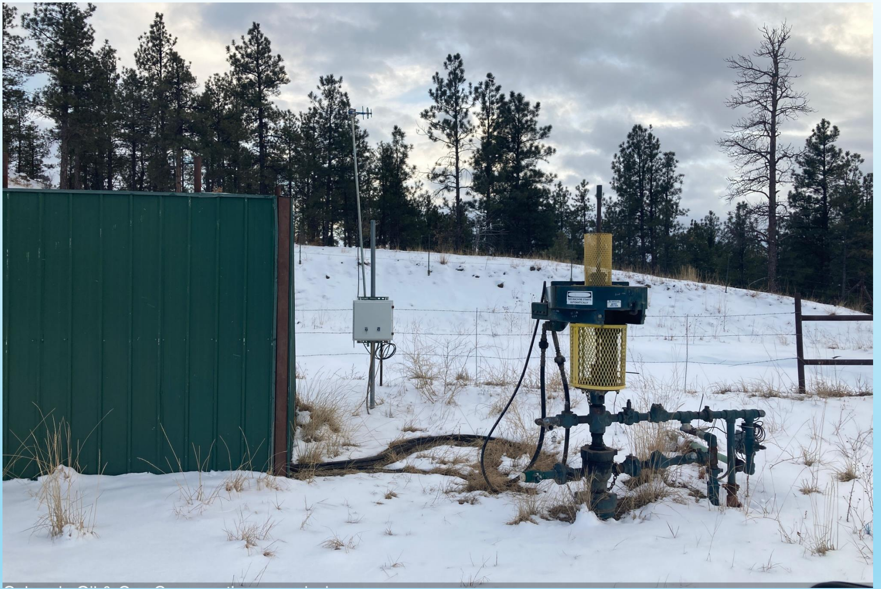
PHOTO 3: WELLHEAD AND EQUIPMENT
