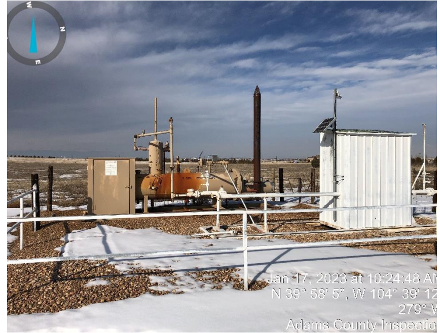
Photo# 2 Separator & Meter house.
