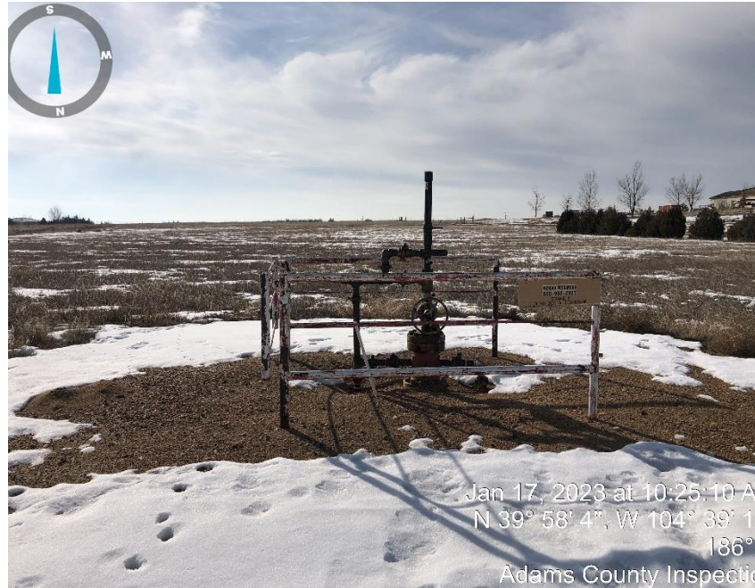
Photo# 3 Well Head.
