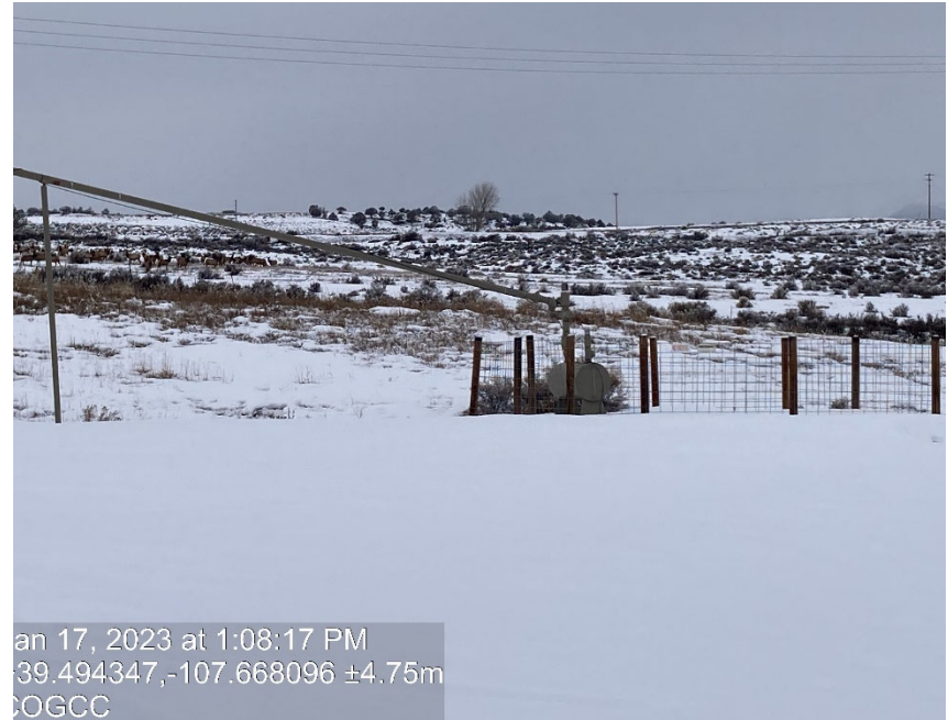
ECD has been removed. Knockout and line from tanks are still in place.
