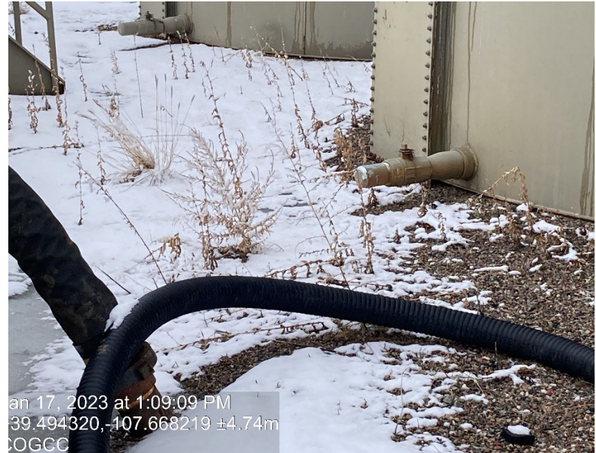
Weeds in secondary containment
