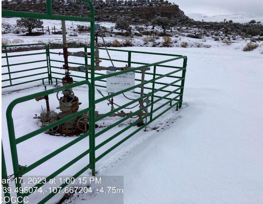
Signage is faded and illegible
