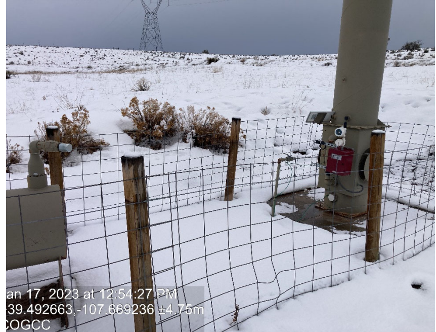
Unused/stored equipment (ECD disconnected)
