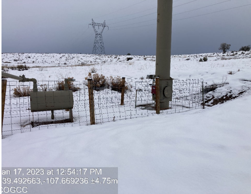
Unused/stored equipment (ECD disconnected)
