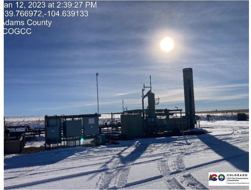
Pic 4 separator, electric equipment, ECD.
