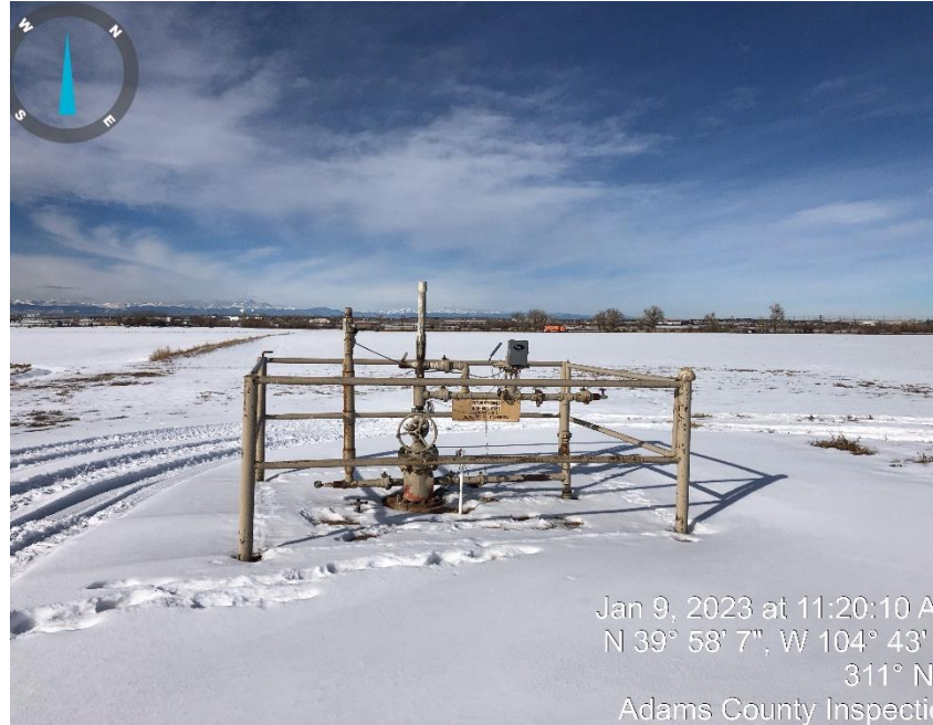
Photo# 3 WELL HEAD.
