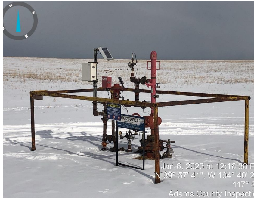
Photo# 3 Well Head.
