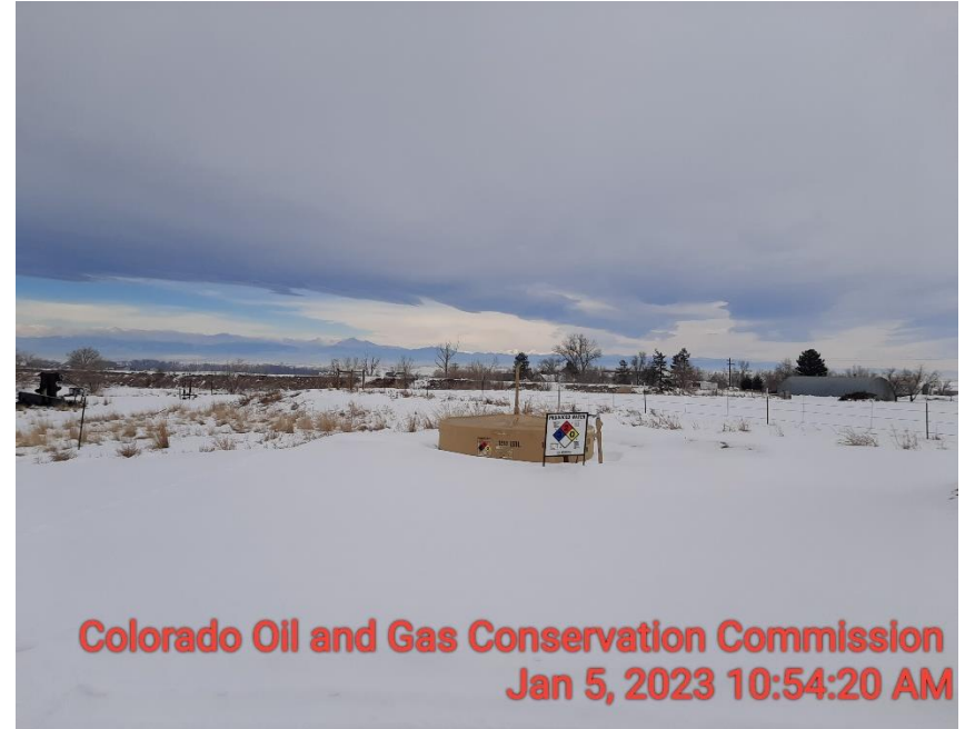
Photo 2 produced water tank
