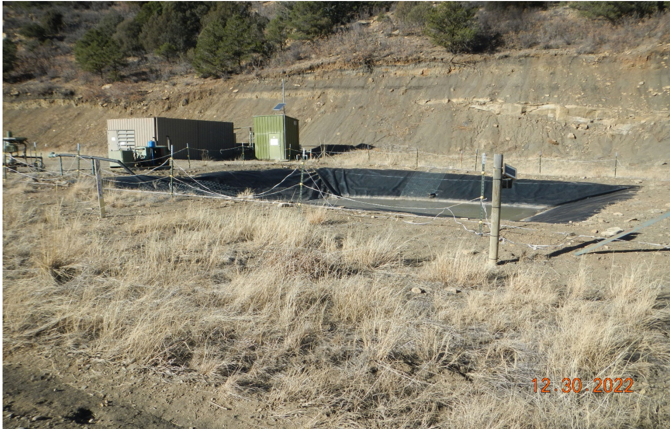
Photo 1. Facing toward the wellsite. The electric fence is in disrepair around the pit. A more robust fencing should be considered.
