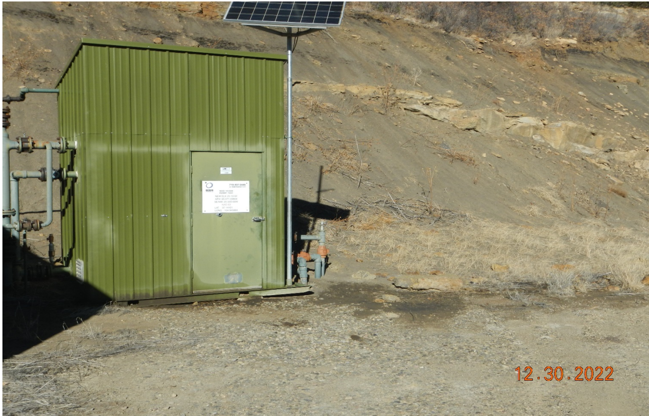
Photo 2. There are stained soils at the meter shed that should be cleaned up and equipment inspected for leaks.
