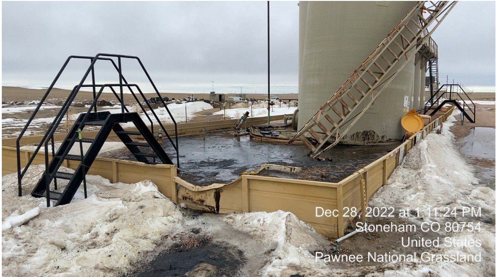
Damaged Produced Water Tank
