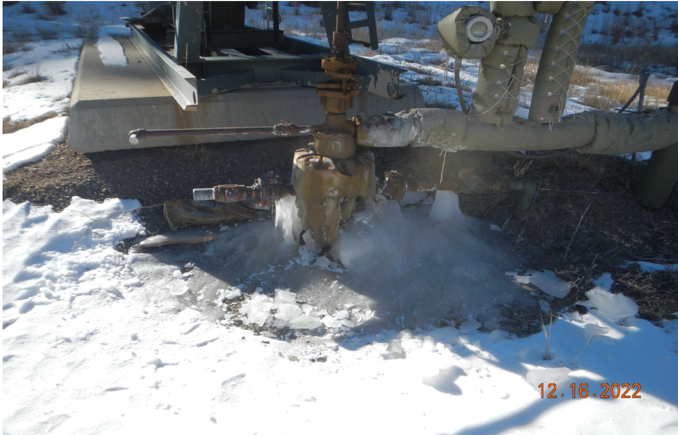
Photo 2. There is ice build up at the wellhead which appears to be leaking.
