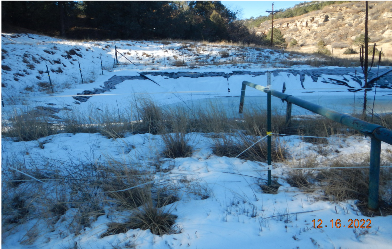
Photo 3. Facing toward the lined pit. The electric fence needs maintenance.
