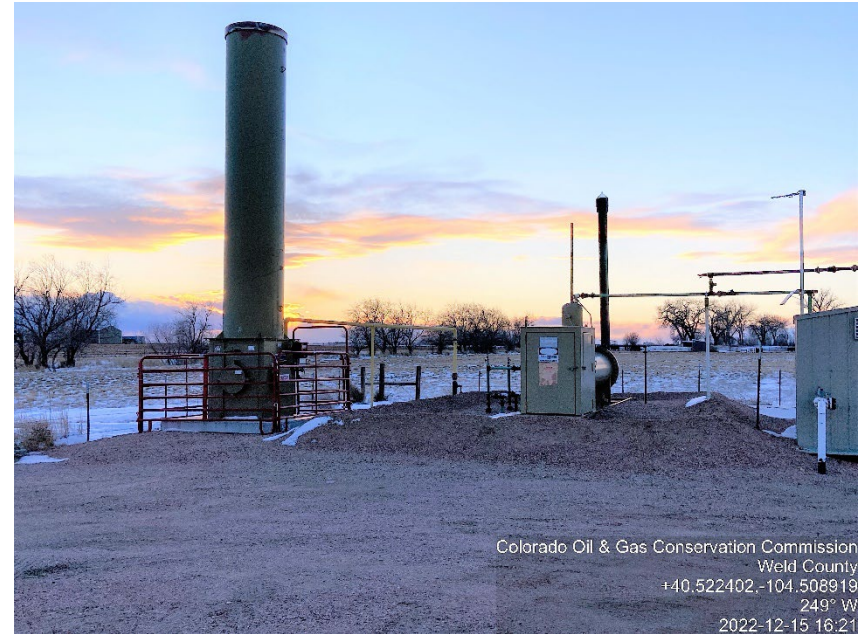
Photo #4 Cecil 41-2, 31-2 Battery site Inactive | Shut-down Separator, ECD
