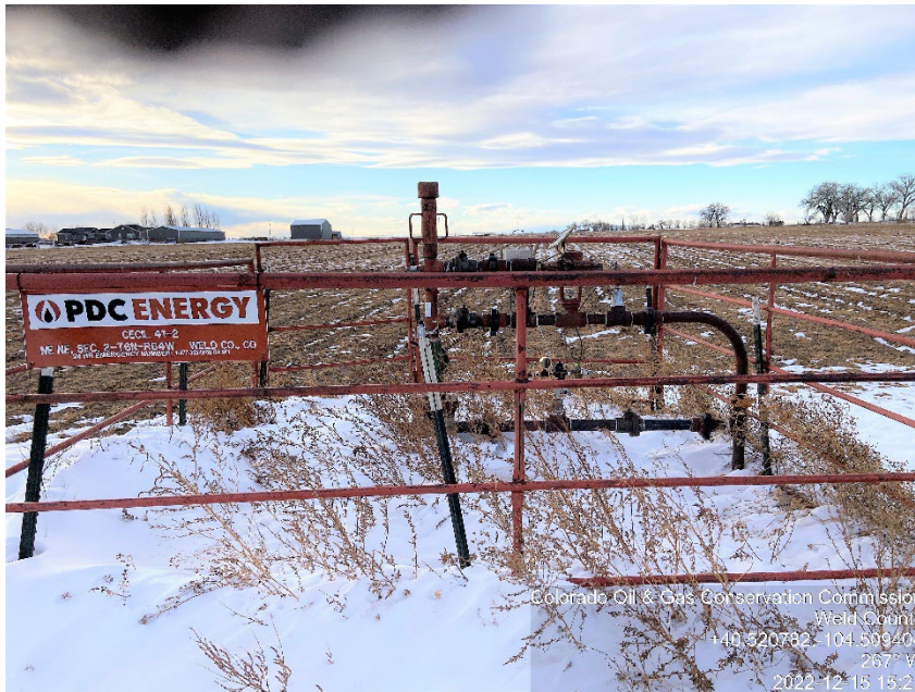
Photo #1 Cecil 41-2 (123-22707) Wellsite Shut-In | SI
