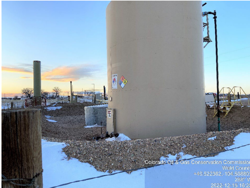
Photo #3 Cecil 41-2, 31-2 Battery site Inactive | Shut-down Tank(s): SE corner
