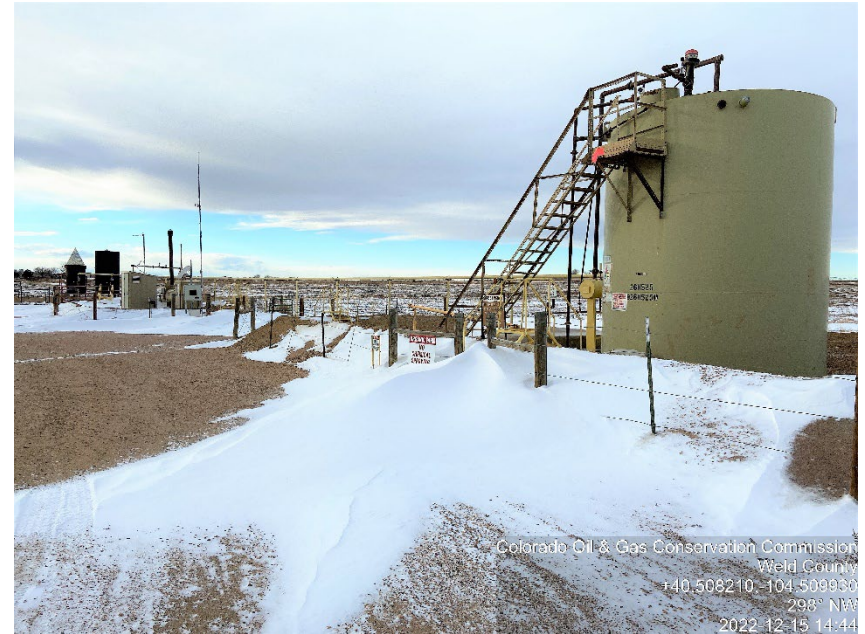
Photo #2 Pettinger 34-2, 33-2, 43-2 Battery site Inactive | Shut-down Formerly served: Pettinger 44-2 ; Plugged & Abandoned | PA Equipment documented: Loc. # 305860
