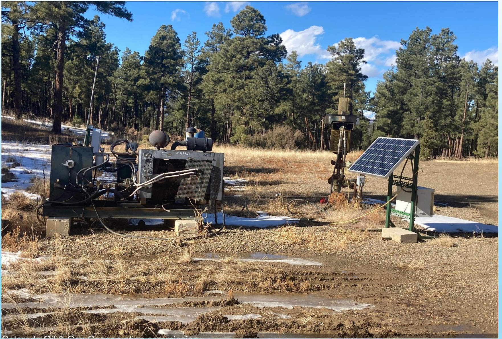
PHOTO 3: WELLHEAD AND EQUIPMENT
