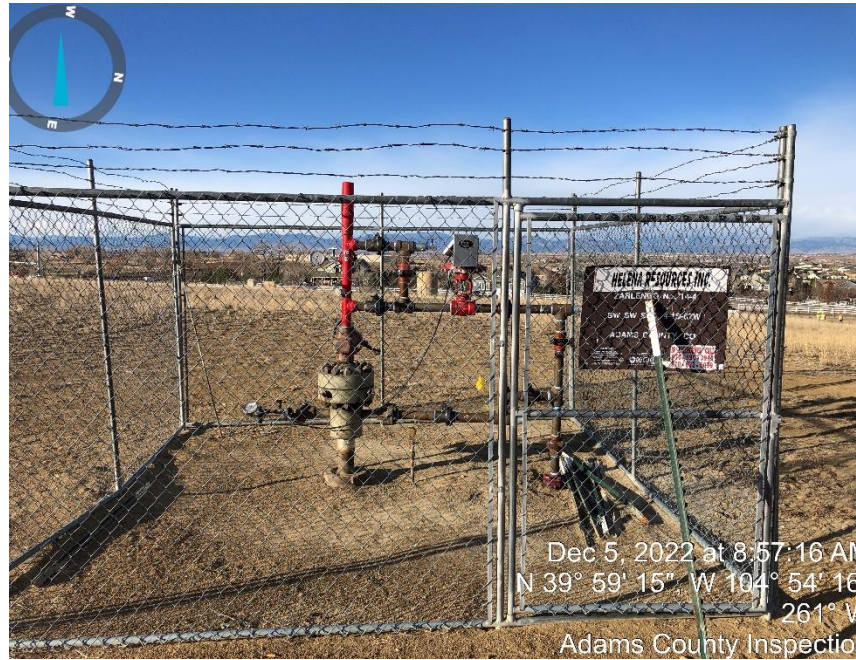
Photo# 3 Well Head.
