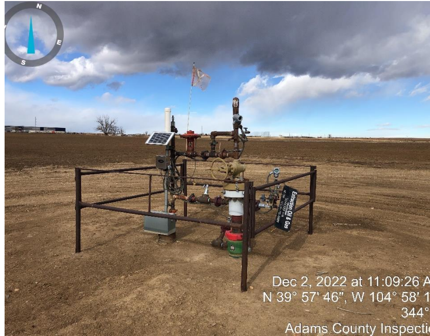
Photo# 3 Well Head.
