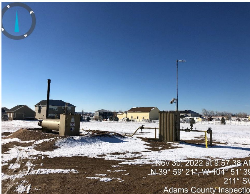
Photo# 3 Separator & meter house.
