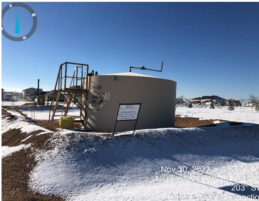
Photo# 1 Crude tank.
