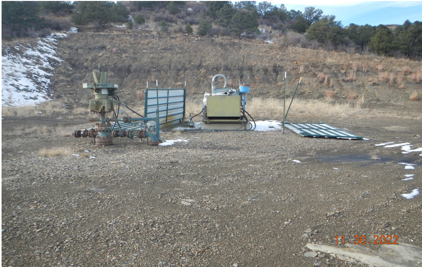
Photo 2. Facing toward the wellsite. There are panel laying on the ground that need to be removed or re-installed.
