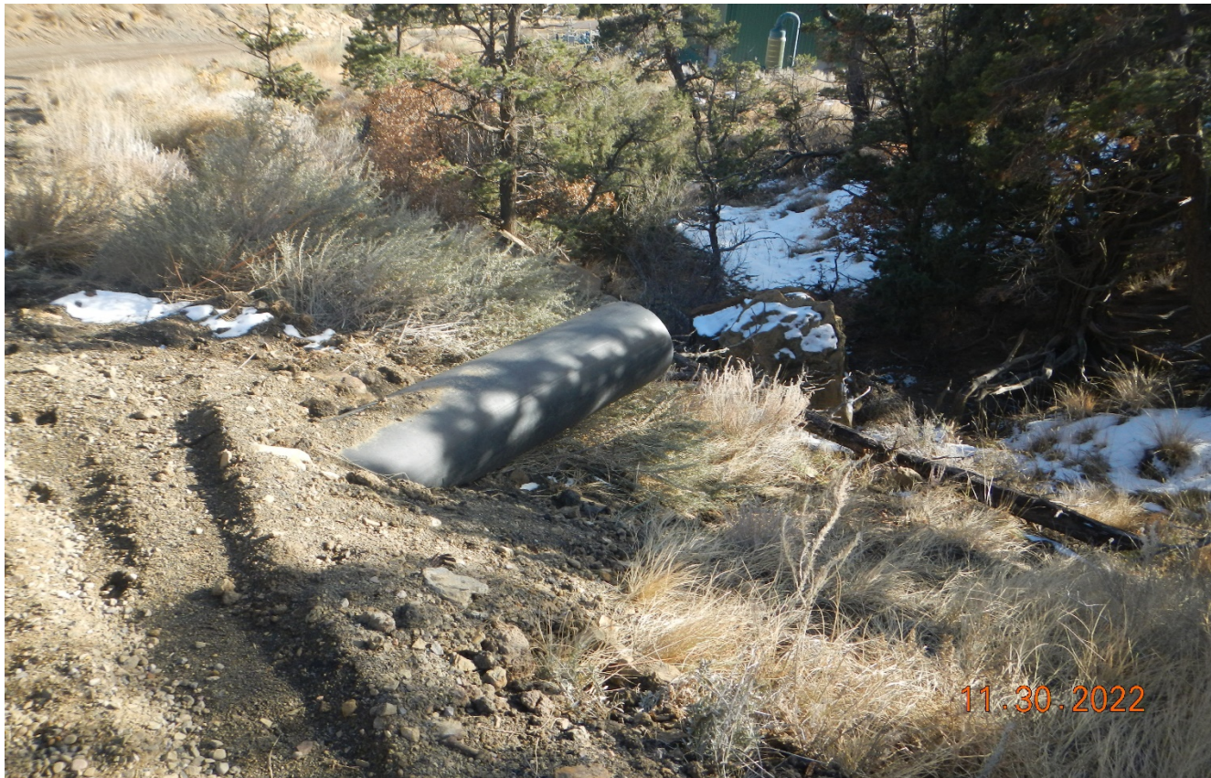
Photo 6. There is no outlet protection installed at the newly installed culvert.
