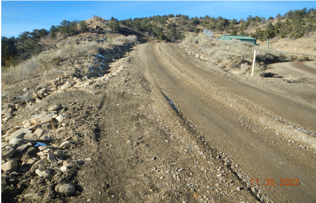
Photo 1. Facing northwest toward the access road. The erosion on the road has been repaired and diversion has been installed off the road side with rip/rap.
