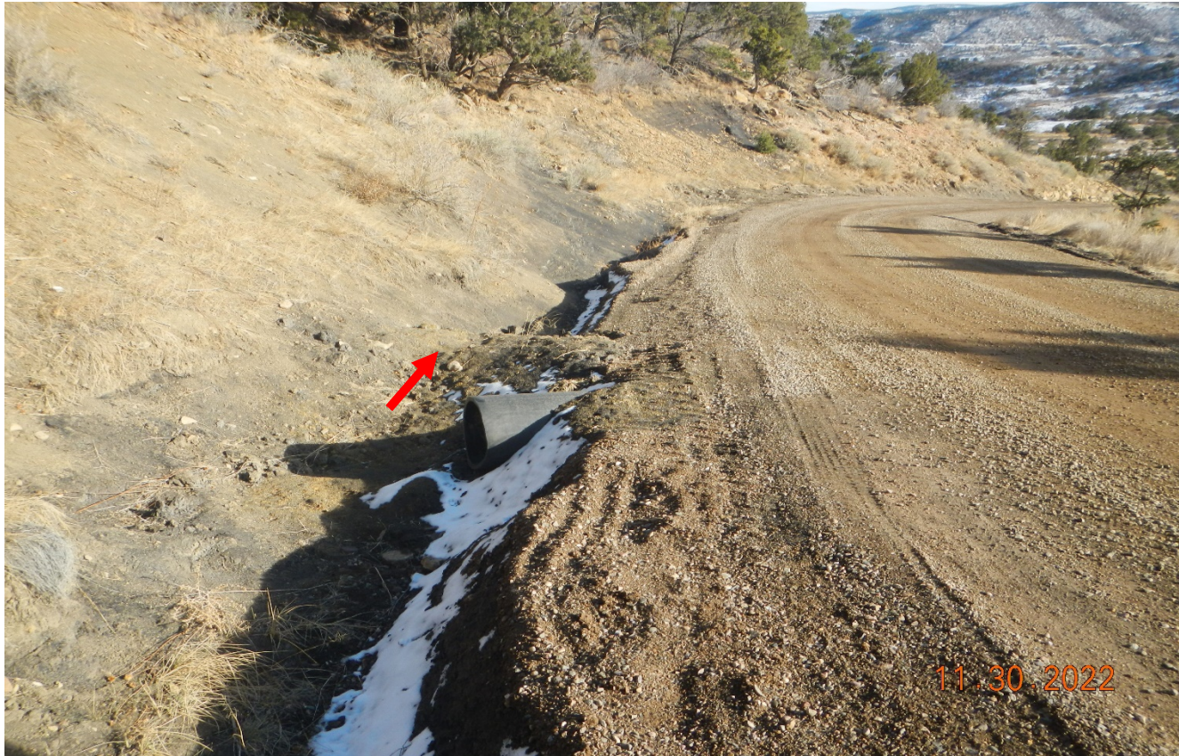
Photo 5. Further up the road a culvert was installed which will help with concentrated flows along this area. There is concerns that stormwater will overtop the embankment at red arrow which should be built up better and compacted.
