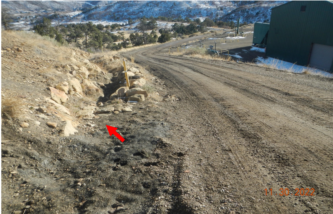
Photo 3. This area along the road may need to be dug out more to ensure stormwater flows into the diversion shown at red arrow.
