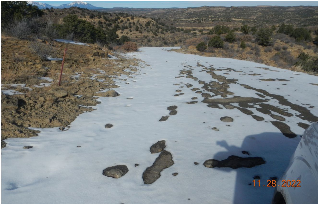
Photo 2. Facing northwest along the access road to the well site. This area of erosion was repaired and stabilized. Snow cover obscures this area at time of inspection.
