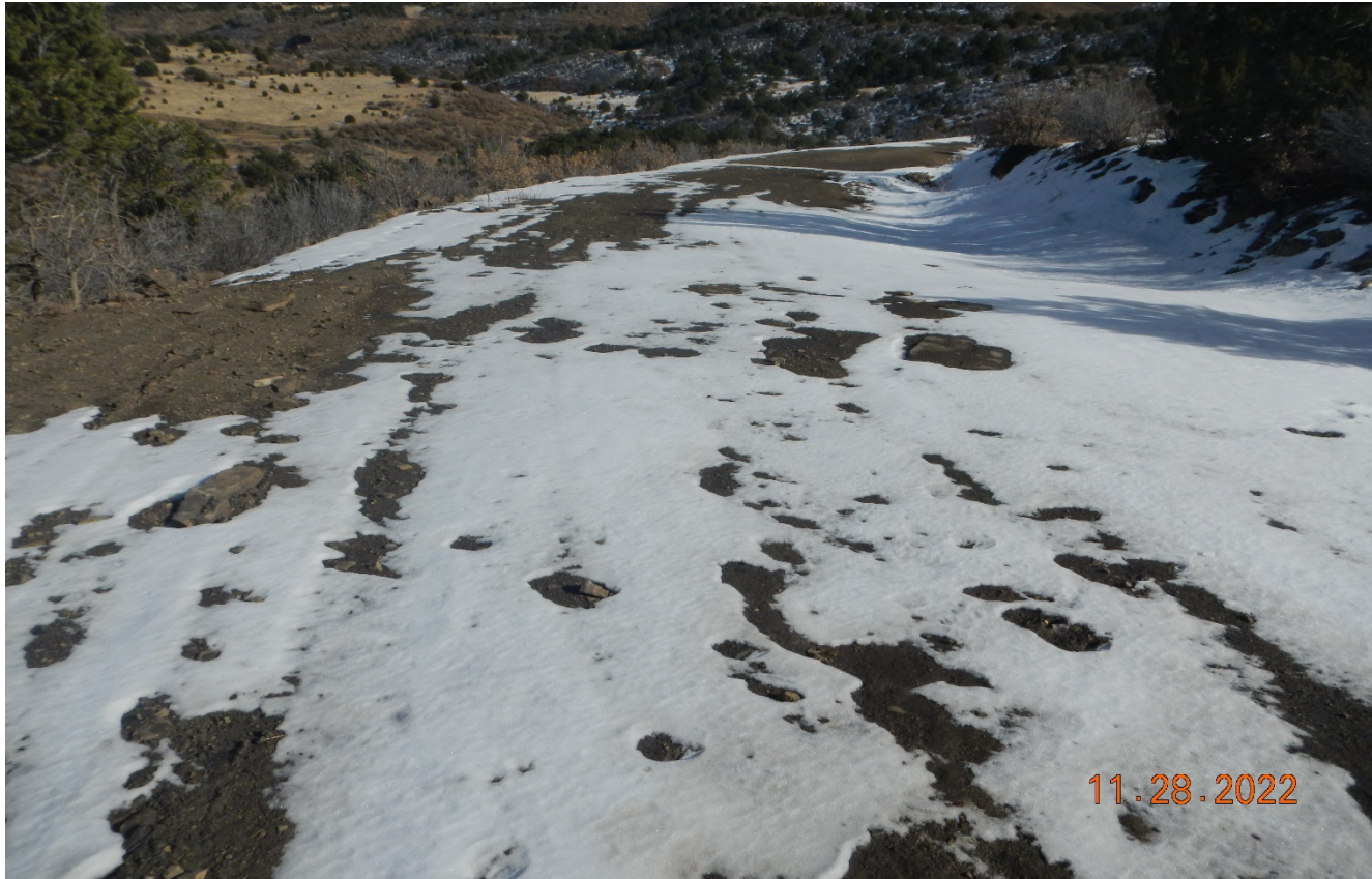
Photo 3. Facing east along the access road to the well site. This area of erosion was repaired and stabilized. Snow cover obscures this area at time of inspection.
