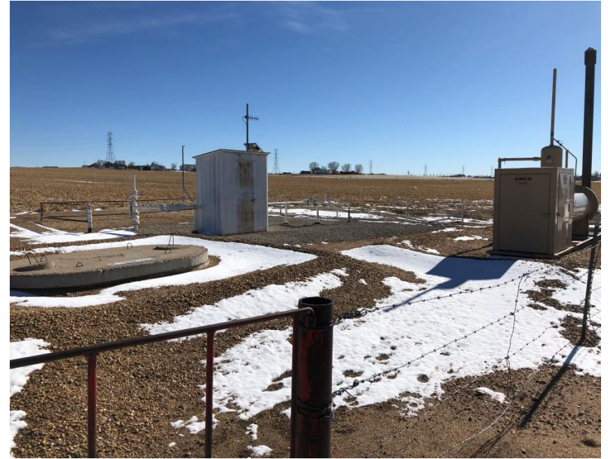
Photo#2 Concrete Vault/Gas Meter/Separator
