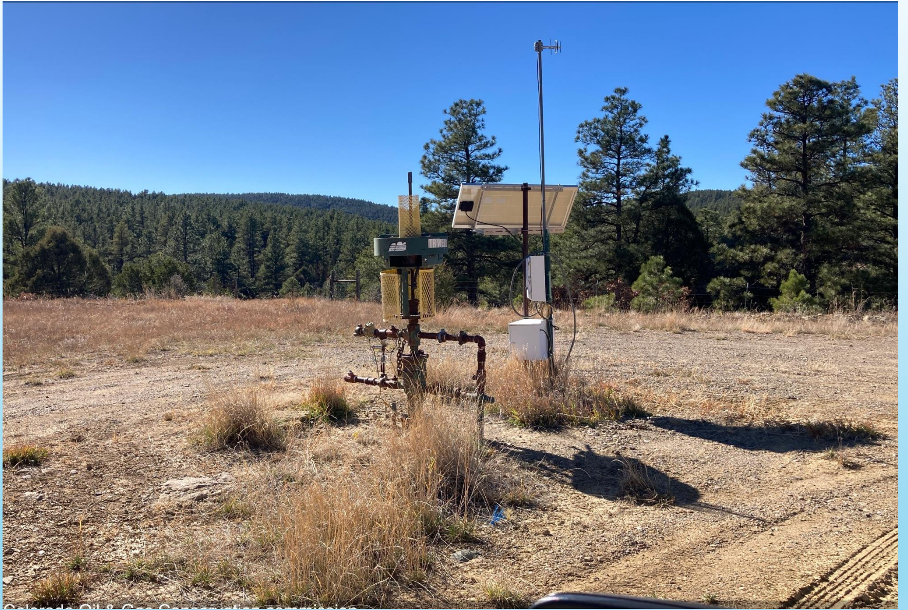
PHOTO 3: TR WELLHEAD AND EQUIPMENT
