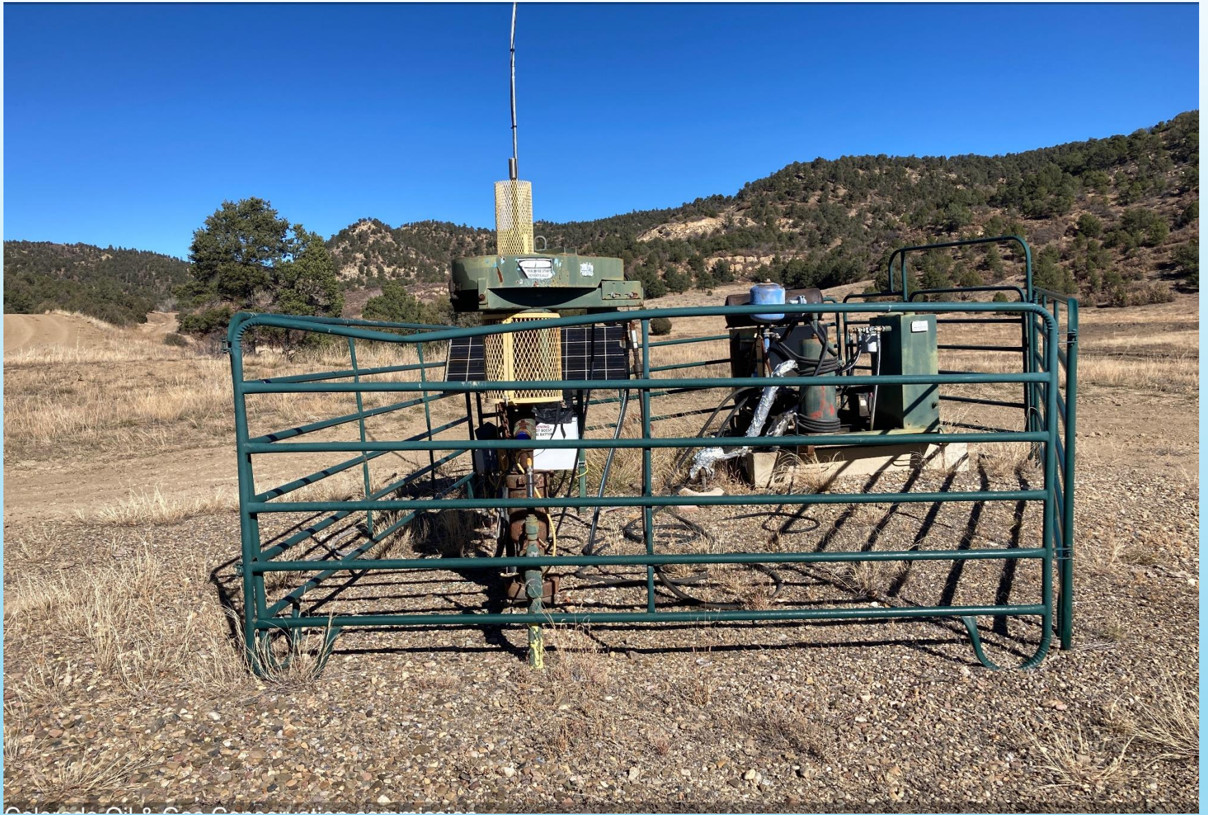
PHOTO 3: WELLHEAD AND EQUIPMENT
