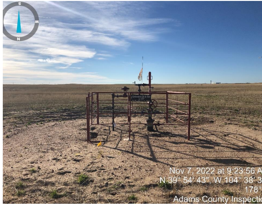
Photo#3 Well Head.
