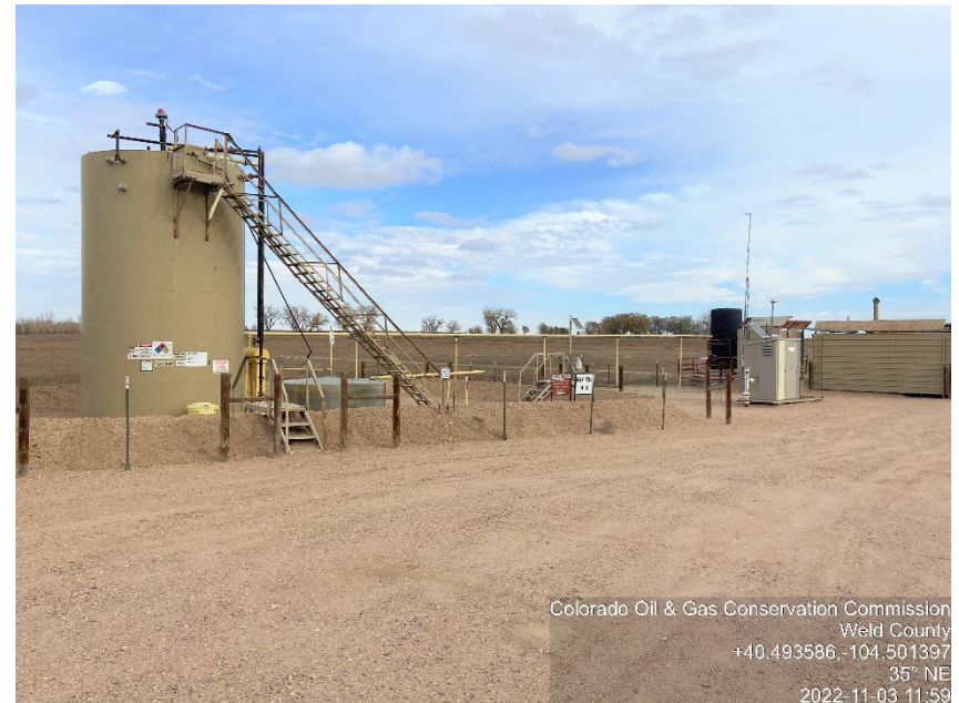
Photo #2 Schant 24-12, 23-12, Lapp 33-12 Battery site Active Equipment documented: Loc. # 332432
