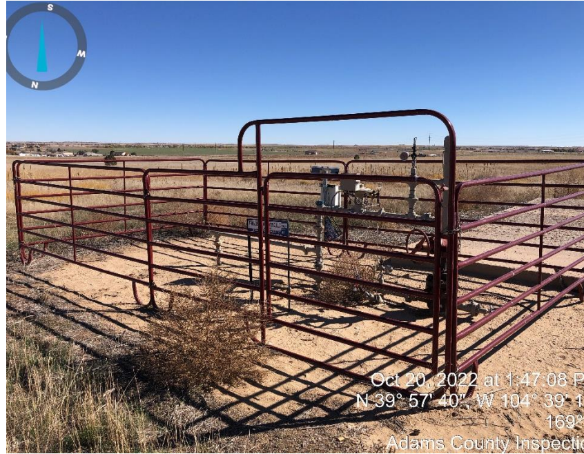
Photo#3 Well Head.
