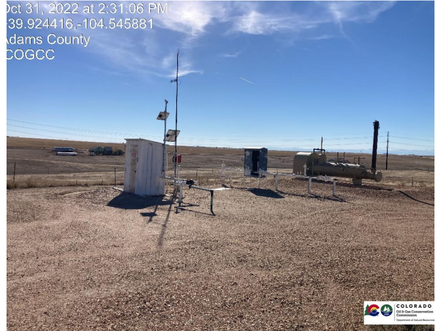
Pic 2 Gas meter runs Separator.
