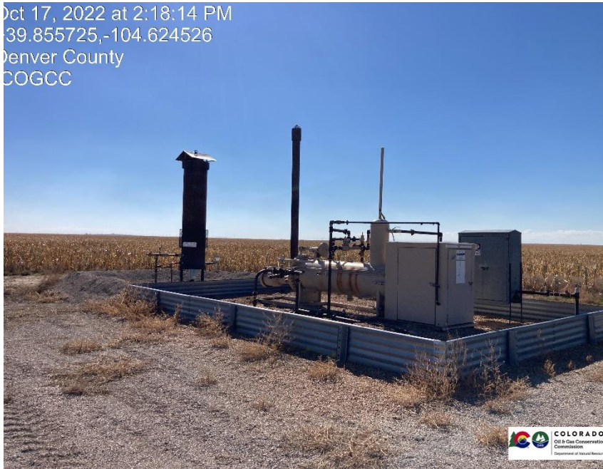
Pic 3 separator, ECD, Gas meter run
