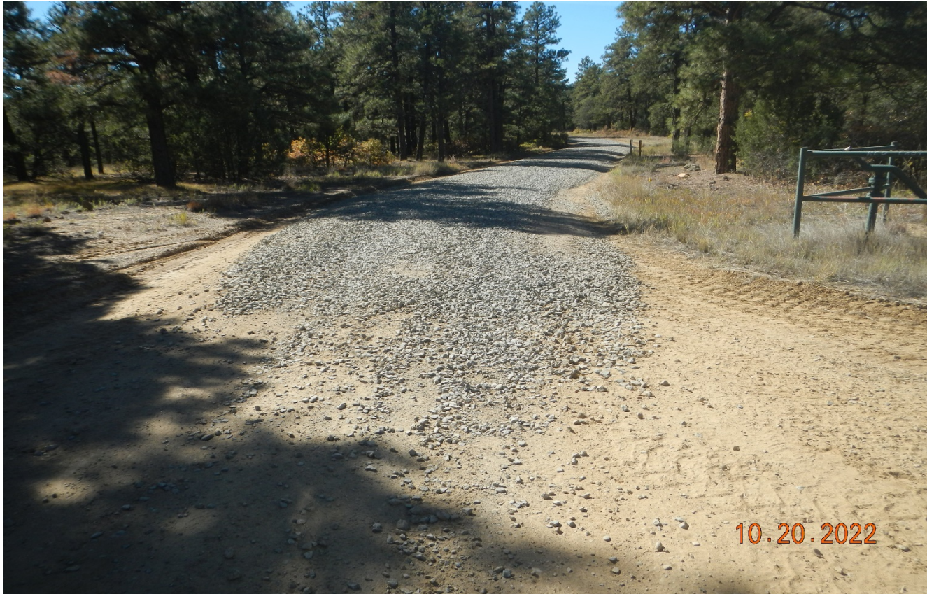
Photo 2. Facing south along the access road. This area of the road has been repaired and stabilized with gravel.
