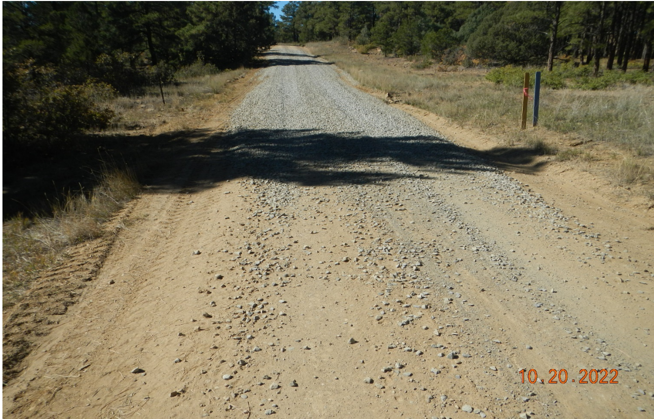
Photo 1. Facing southwest along the main road traveling to the location. This area of the road has been repaired and stabilized with gravel.
