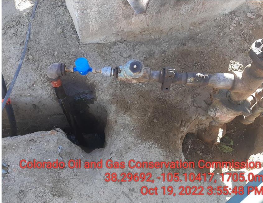
Photo 5 Flow line leaking crude oil from ½ line to well head. Stained soil around well head
