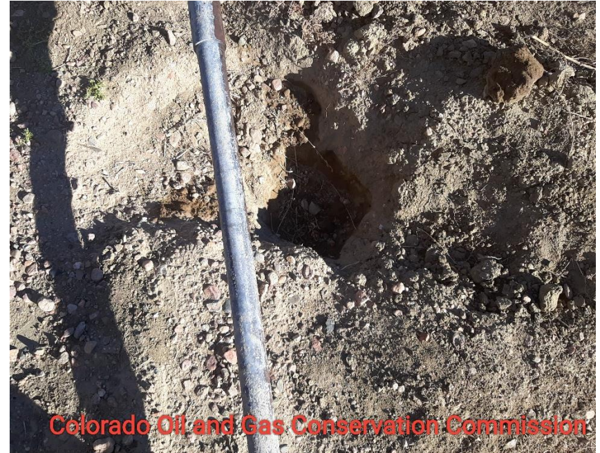
Photo 6 open hole inside unused crude oil tank containment it appears the hole is 10 deep and has stained soil .
