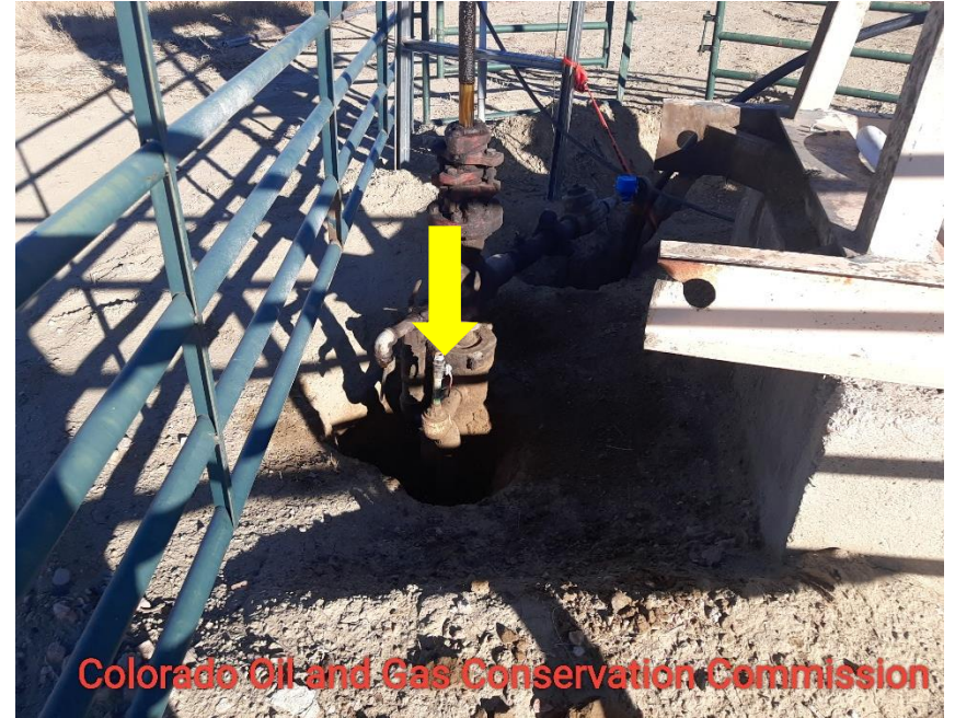
Photo 8 Well actively venting gas through 1/2 line off well head is open.
