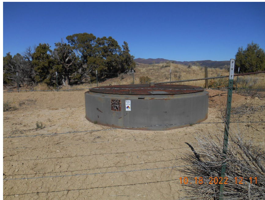
Produced water tank battery
