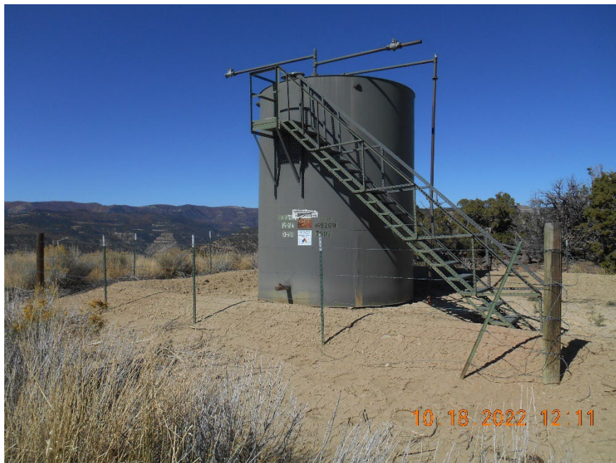
Crude oil tank battery
