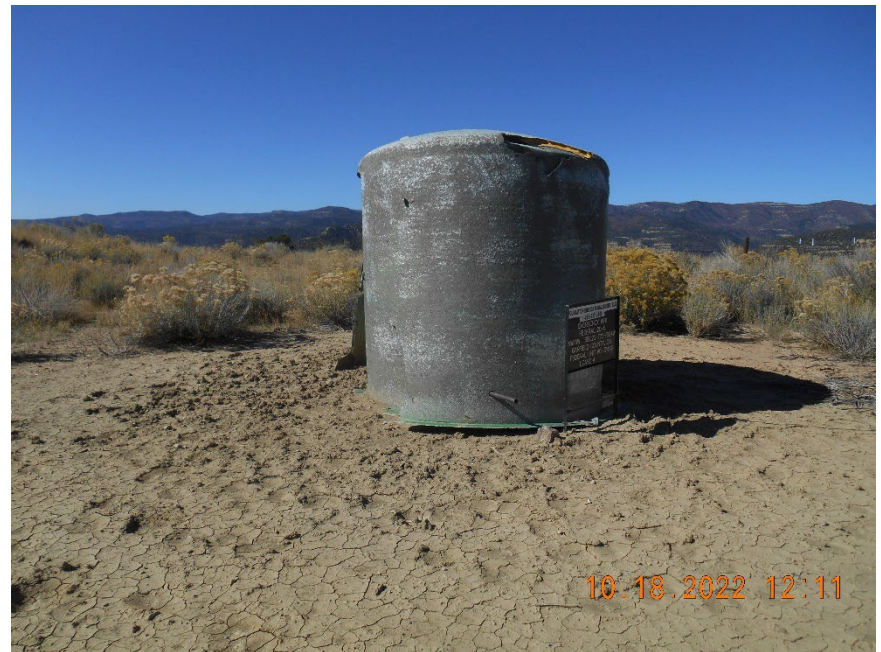
Wellhead inside fiberglass housing
