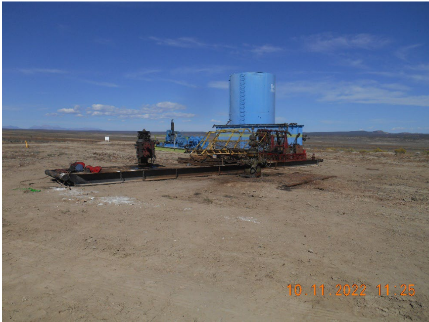
Wellhead with remaining workover equipment.
